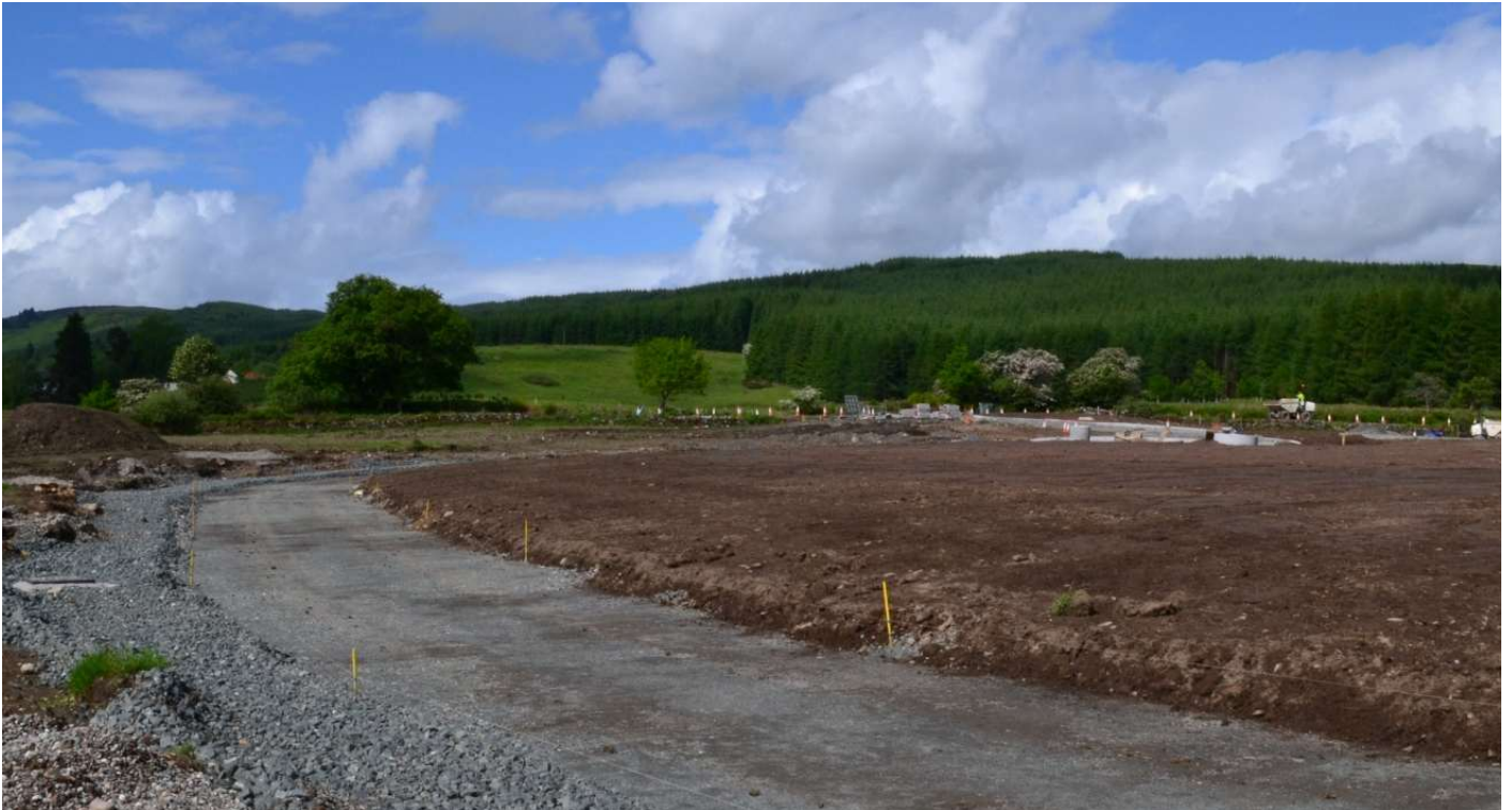
Figure 8. Early works at the new Balvalachlan cemetery near Callander, Scotland. The young oak near the centre of the image was initially marked for removal but retained during construction, becoming part of the site's future memory and long-term character. Photograph by the author, 31 July 2018.
